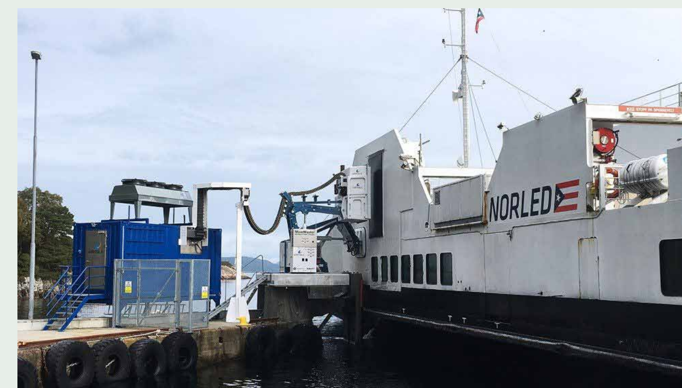
Fig. 3 Wireless inductive charging (Photo: Wärtsilä)
